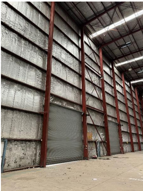
I14-01 Source p.14 top-left Roller shutters and personnel door interrupt the wall; header, jamb and brace relationships.
