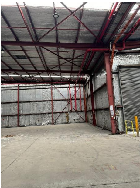
I11-06 Source p.11 bottom-right Overhead/vertical runs, fittings and wall opening. Contents and status require records.
