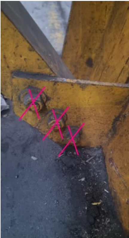
Original report p.22 Fig.7. Source marks identify a connection review location. They do not establish the current residual stability.
